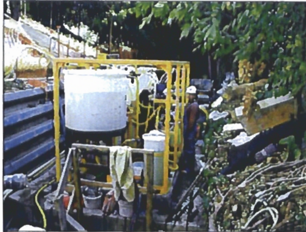
Figure 4. Sodium silicate grout plant.
